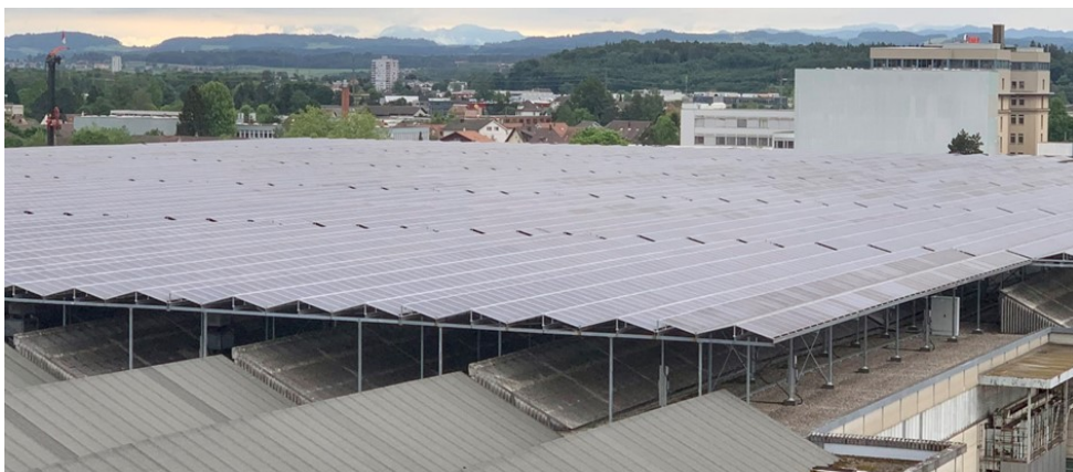
PV Anlage Riverside
